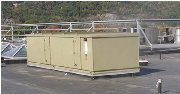
Trane rooftop AHU installed
